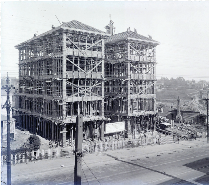
Figure 15. "Mayfair Residential Flats on Parnell Road Under Construction." Published in the Auckland Star , 20 September 1928. Photographer Unknown. Auckland Libraries Heritage Collections 1285-10011. Note the very deep concrete beams at each floor level of the front elevation.
